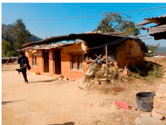
Fig. 3. Damaged house in the study area after the earthquake.
